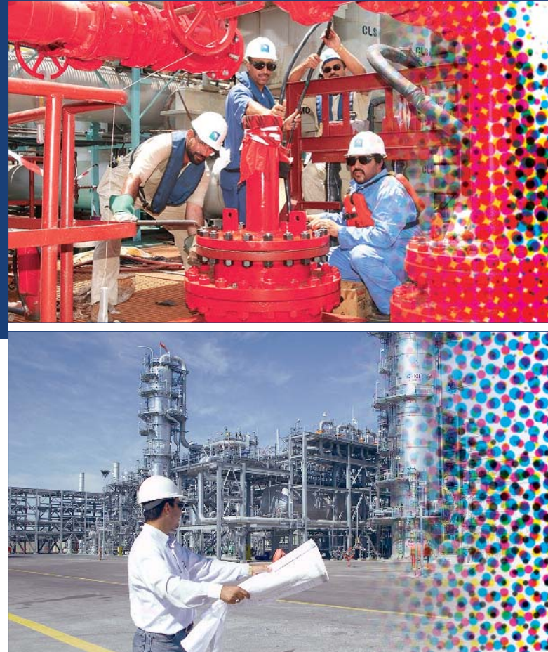
Top: Workmen secure new pipe connections at Ras Tanura Refinery. Above: An engineer inspects a process unit.
